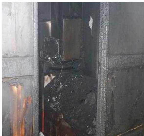
<Photo 2> Inside room no. 6, the suspected point of origin
