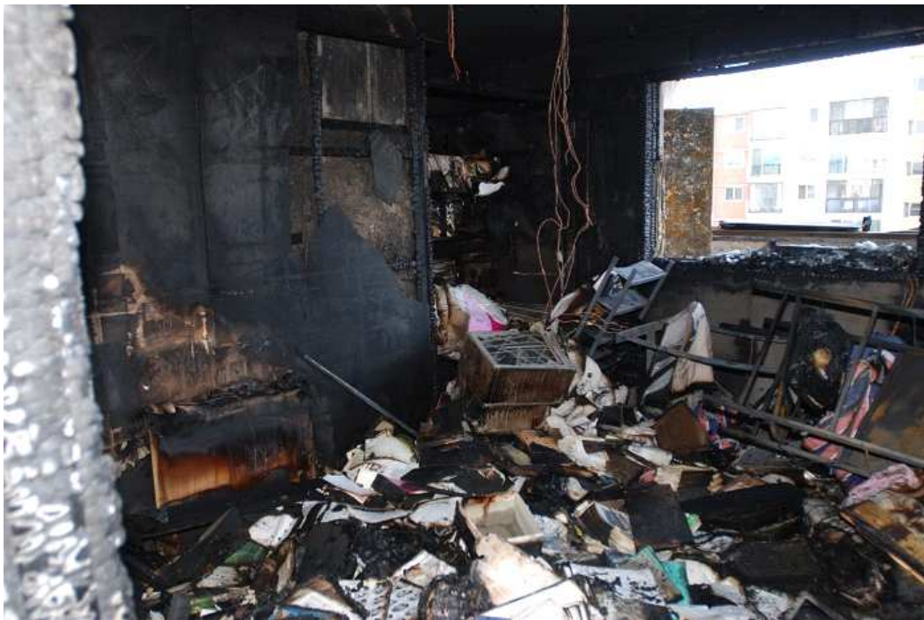
<Photo 2> Small room, the point of origin
